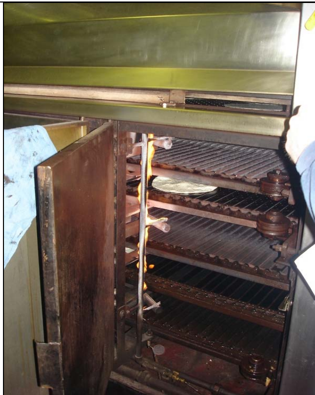
THREE TIERS: BURNERS LEFT SIDE/ NOZZLES MOUNTED RIGHT SIDE
