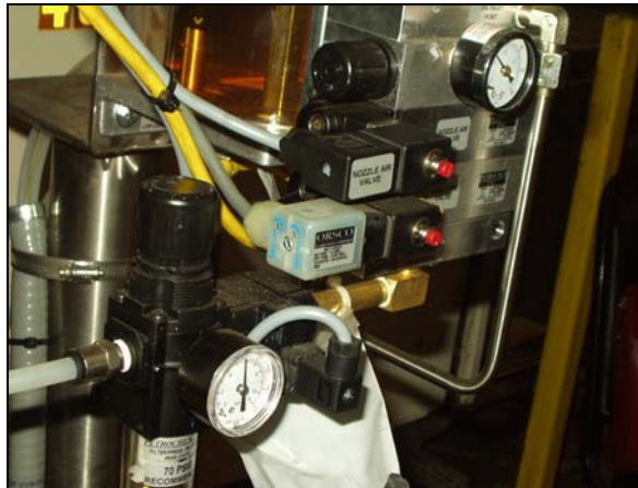
NOZZLE AIR VALVE & INJECTOR VALVE
